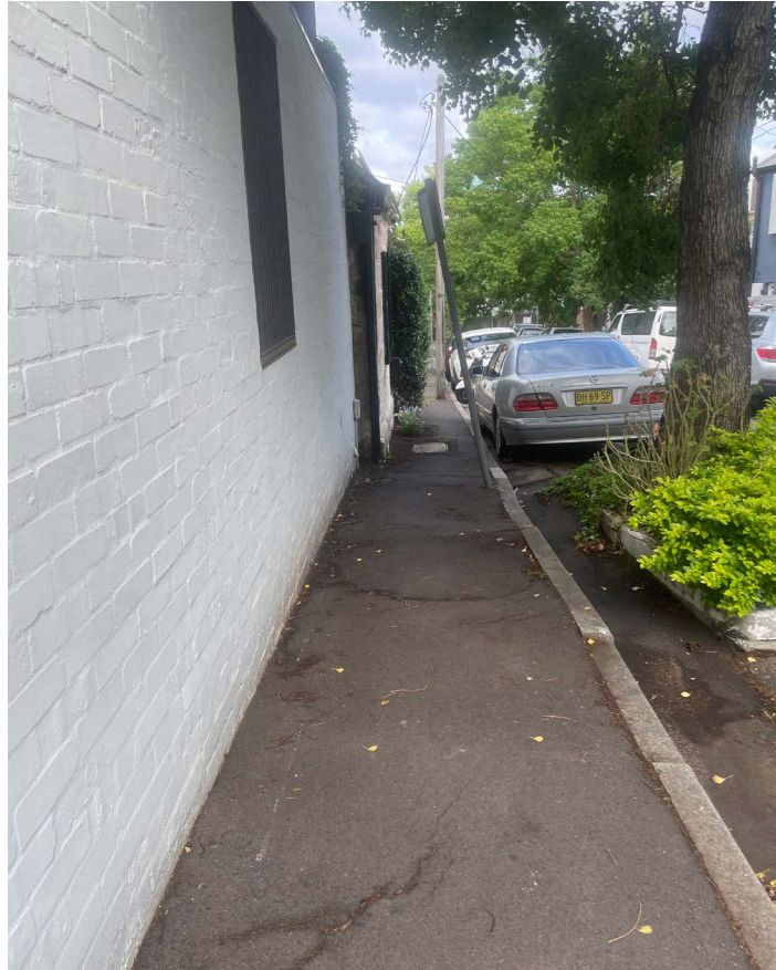
Cracked and narrow pavements on Gipps Street, taken from Shadforth Street corner.
