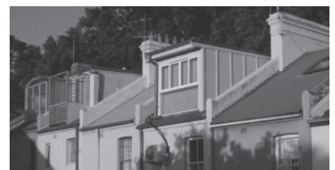
Dormers: CoS DCP don't meet heritage standards
